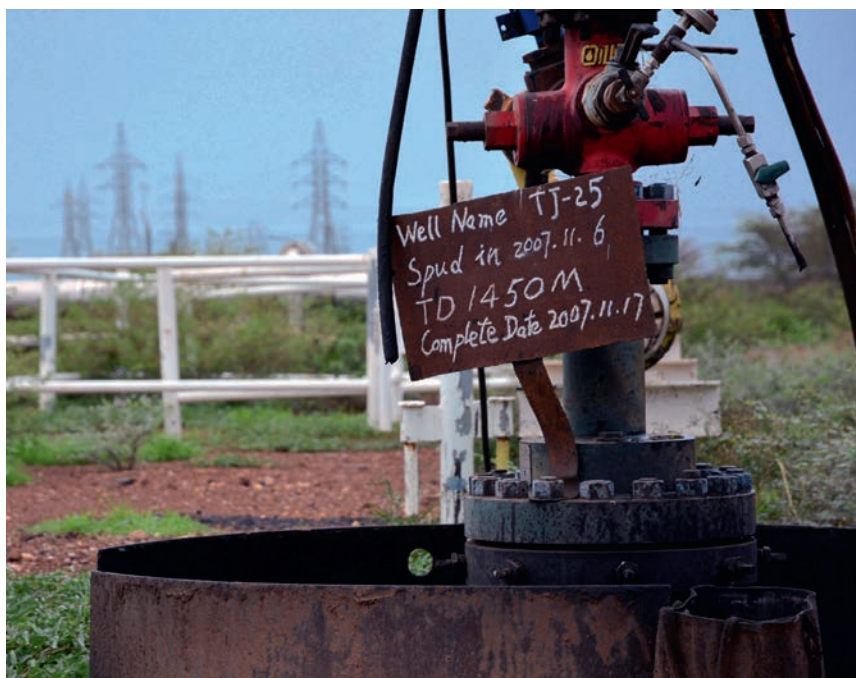
A well and electric poles of the Thar Jath oil fields. All of Unity state's oil installations were shut down days after the new war started in South Sudan, in December 2013. © Jérôme Tubiana
